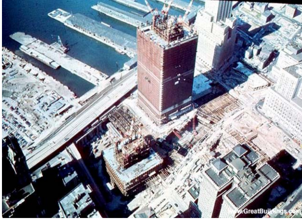
Figure 2: World Trade Center tower being built in 1971. A failed butterfly spandrel support structure was investigated for its future integrity.
